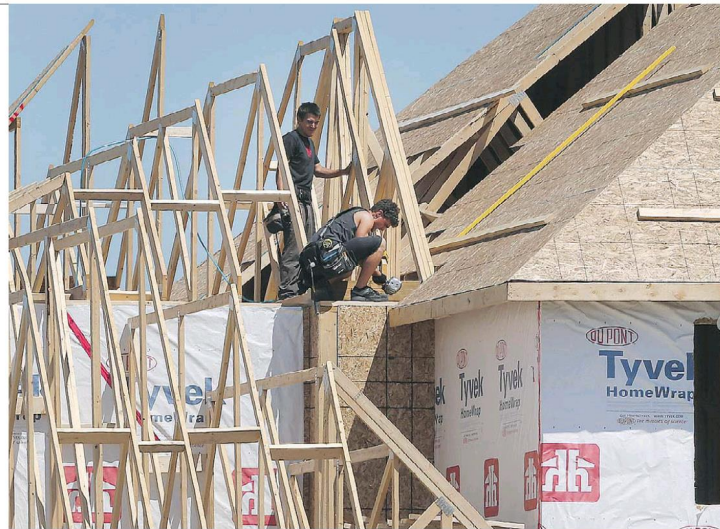
Framers work on a new home on Ryan Avenue in Lakeshore on Thursday. The municipality issued 141 house permits over the first five months. DAN JANISSE
